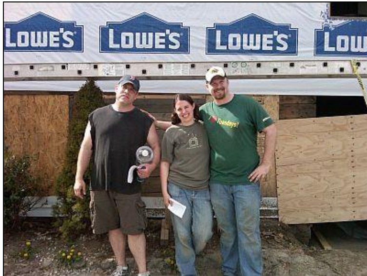
Construction Volunteers enjoy their day with Habitat working at 32 Carter Street in Lancaster.
